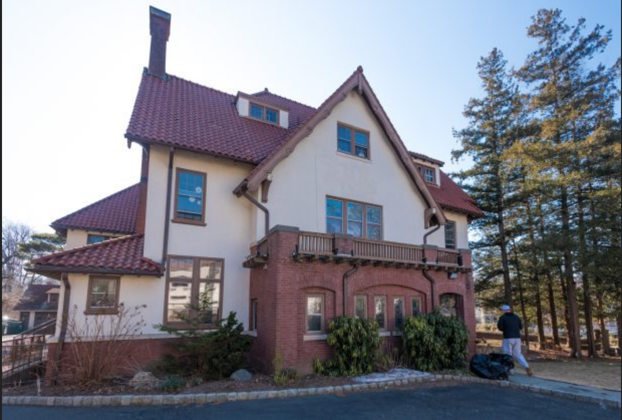
The Montclair Sanctuary Project at Bnai Keshet, a team of about a dozen volunteers from a variety of religious institutions complete repairs and painting Saturday Feb. 3 to the third floor of "Red Gables" at Bnai Keshet, a shelter for immigrants in danger of deportation. ADAM ANIK/FOR MONTCLAIR LOCAL
