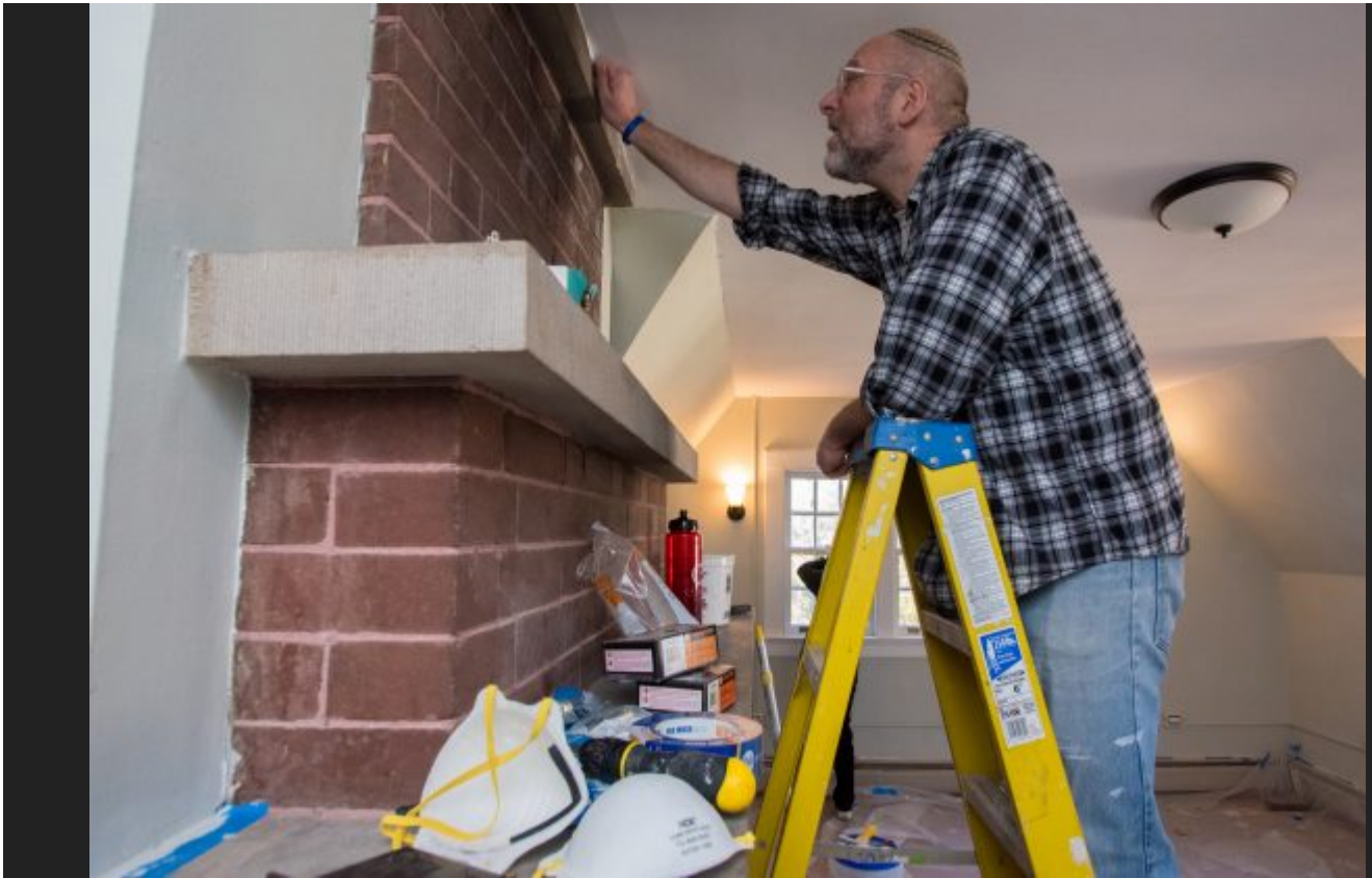
Jordan Sklar of Bnai Keshet cleans paint from the fireplace in the living room in Red Gables on Saturday Feb. 3. ADAM ANIK/FOR MONTCLAIR LOCAL
