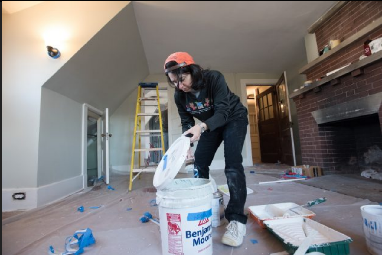
Co-organizer Melissa Polaner of Bnai Keshet mixes paint to be used for the third floor of Red Gables, a shelter for immigrants in danger of deportation. ADAM ANIK/FOR MONTCLAIR LCOAL
